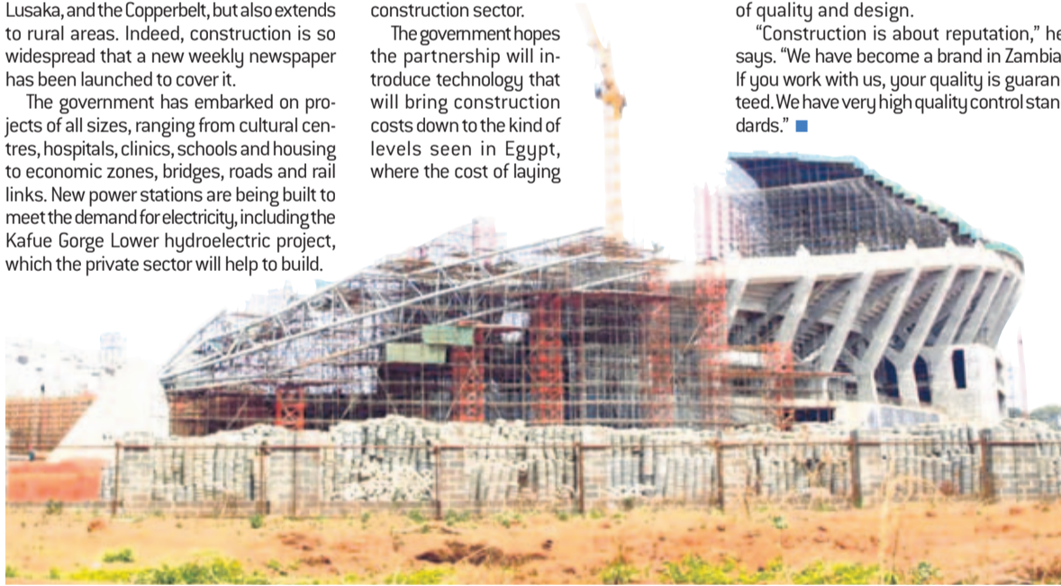
Zambezi Portland Cement is providing critical cement supply for Chinese contractor AFECC's construction of the Ndola Football Stadium
